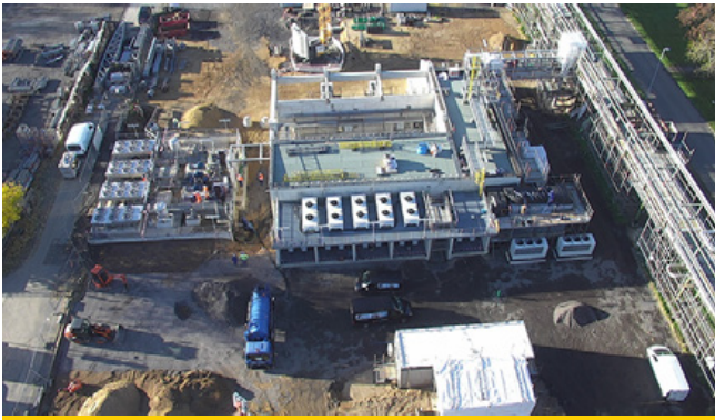
SESCo discussed the new hydrogen electrolyser project at Shell's Rheinland refinery in Germany as part of a virtual site visit.
