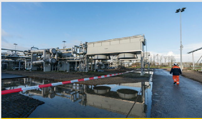
NAM continued to decommission its gas production facilities in Groningen in 2020.
