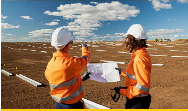
The Gangarri Solar Project in Australia will help power our QGC natural gas project in Queensland and has the potential to reduce QGC's carbon dioxide emissions by around 300,000 tonnes a year.
